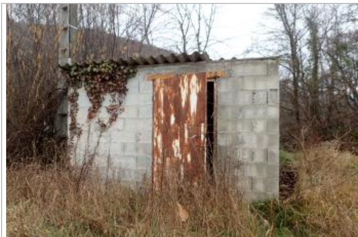
Local pompage - Photo ©AGERIN
