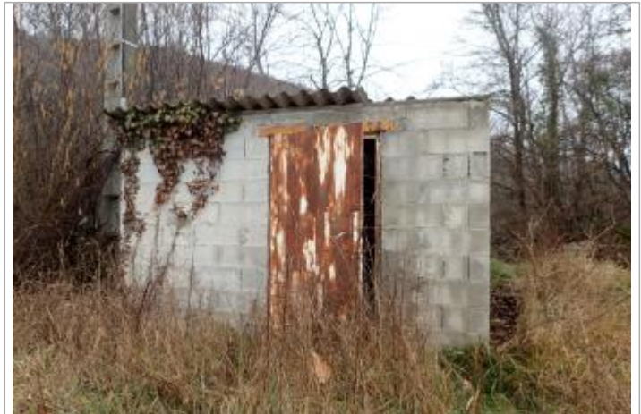
Local pompage - Photo ©AGERIN
