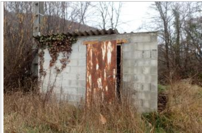
Local pompage - Photo ©AGERIN
