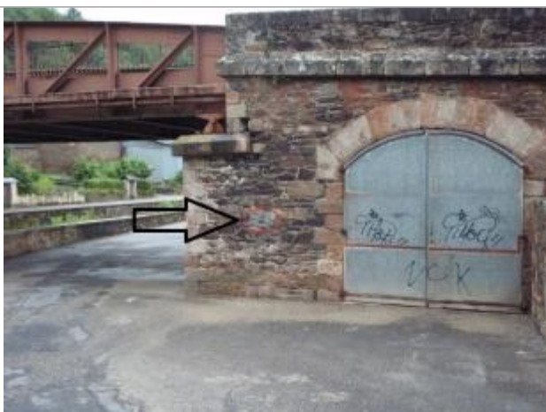
Photo © EPAGE VIAUR
