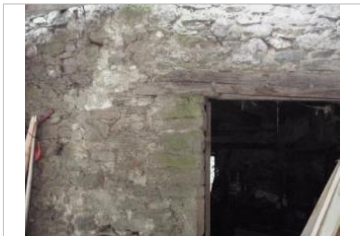
Photo © EPAGE VIAUR
