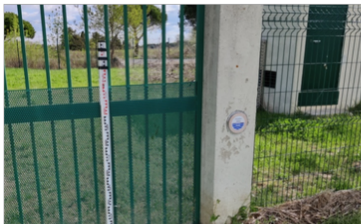
pilier station pompage
